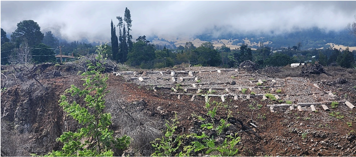
Figure 15. Upper Kula erosion control using eucalyptus logs and wattle chips above the gulch.
